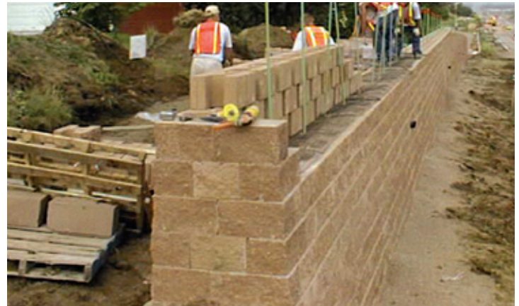
The geotechnical engineer specified gravel fill rather than concrete for this barrier wall made of back-to-back modular units so that it could be more easily repaired in the event of an accident.
