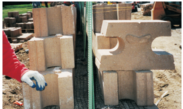
Vertica® retaining wall system blocks in the barrier wall were tied together with geogrid reinforcement.
