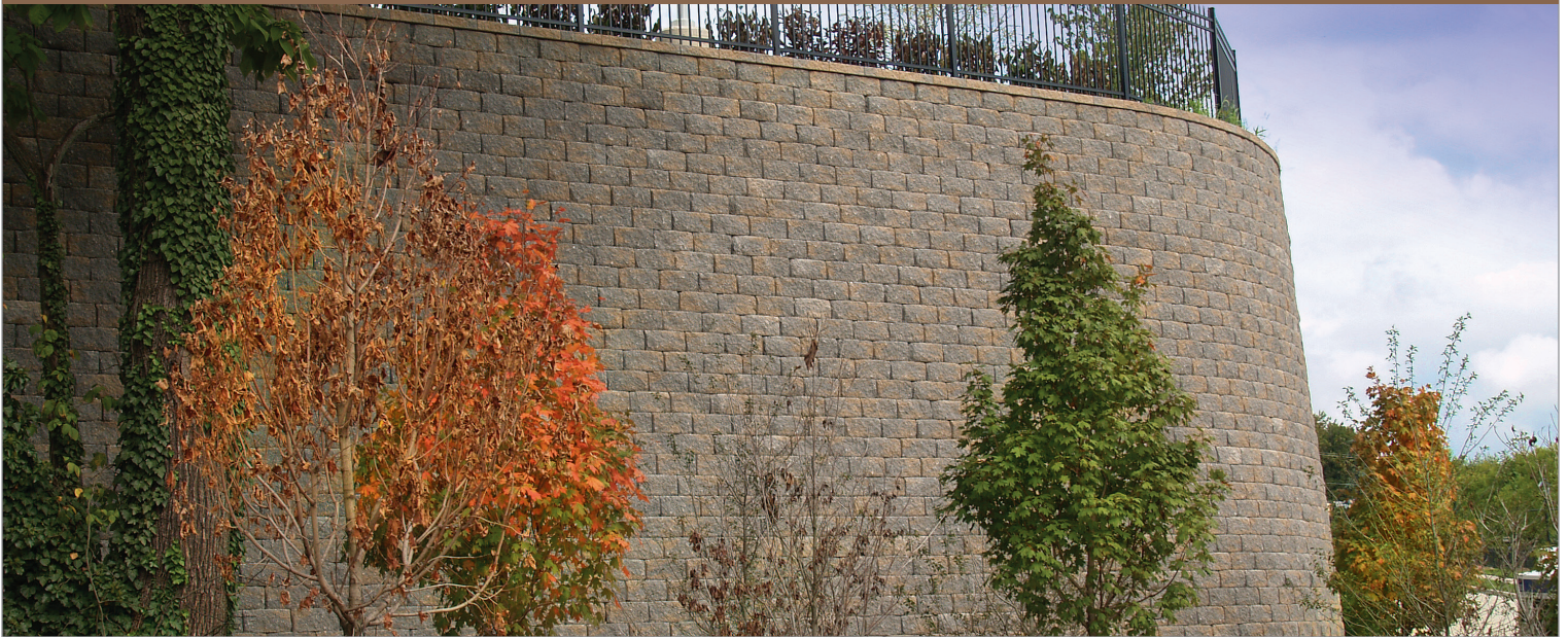
A car dealership added a needed parking lot by using the Vertica Stone Cut® retaining wall system.
