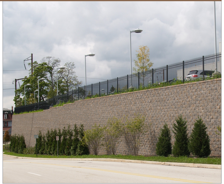
This site was an unusable slope before a retaining wall shored up the site to support a parking lot.
