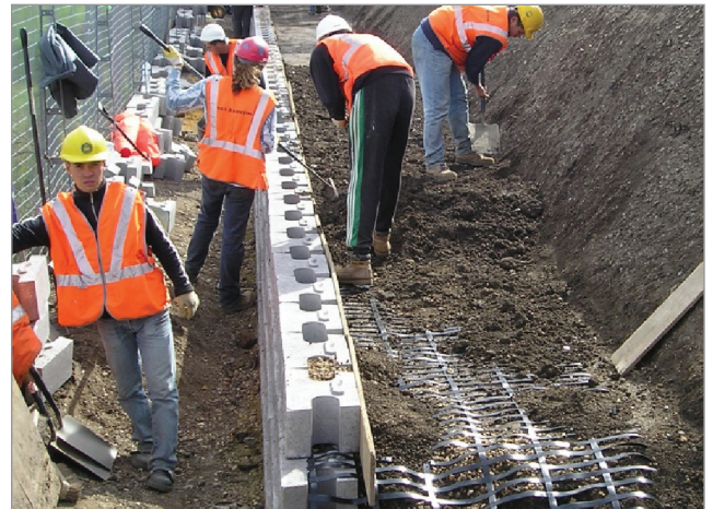
Construction crews installed geosynthetic reinforcement at the bottom of a 45-degree slope and in a space with little room to stage product and work.
