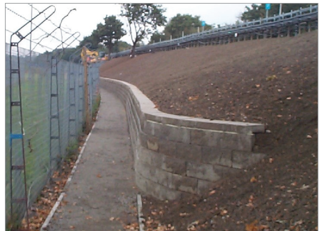
The completed wall provides stability and a pleasant-looking retaining wall for the adjacent residential property.
