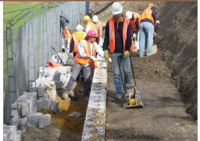
The Vertica® retaining wall system was the right choice for a tight workspace near London, England.
