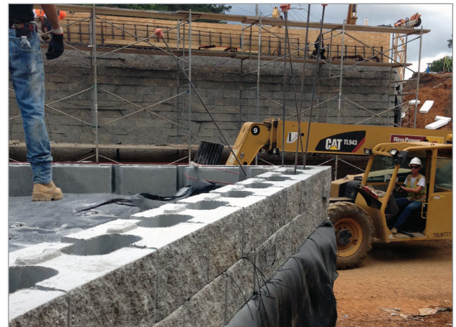
Special cuts in the Vertica® wall blocks were reinforced with rebar for the acute abutment walls.
