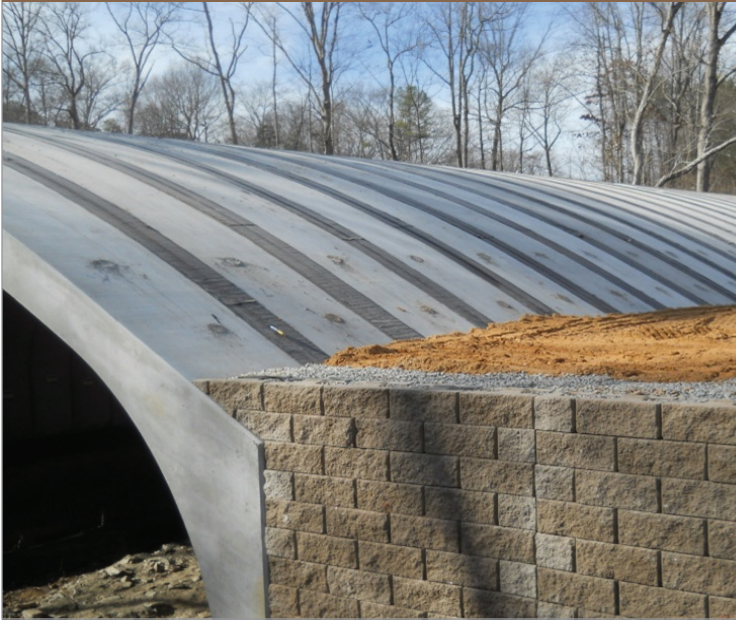
Bridges were constructed with massive, 50-foot-wide arch culverts and the Vertica Stone Cut® retaining wall system.
