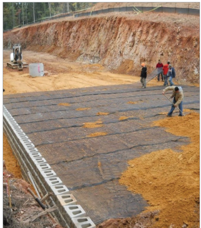
Most of the onsite soils weren't suitable for retaining wall construction.
