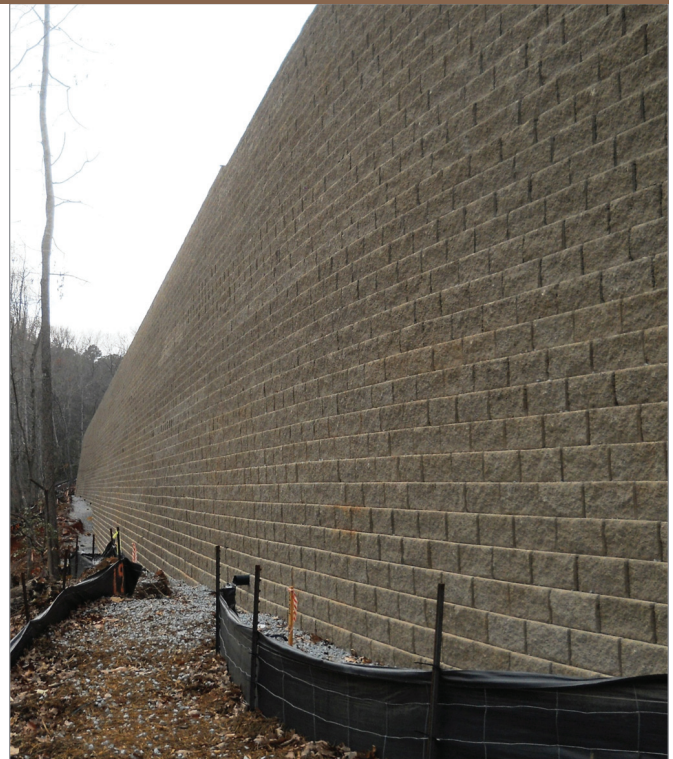
One of the first walls built was a 48-foot-tall (30,000 sq. ft.) Diamond Pro Stone Cut® retaining wall.
