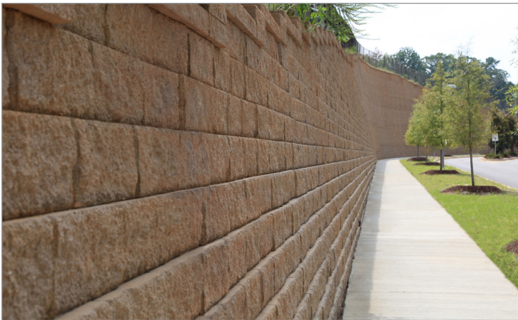
The primary use of the walls was site preparation but the finished walls received praise for overall appearance.
