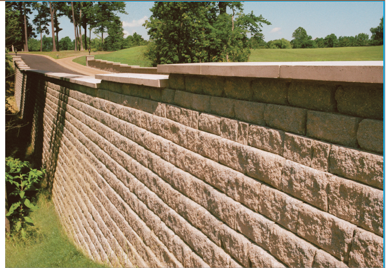
The land bridge utilizing Diamond Pro Stone Cut® and Highland Stone® retaining wall systems, combined with the load-transfer platform, offered 50 percent cost savings.
