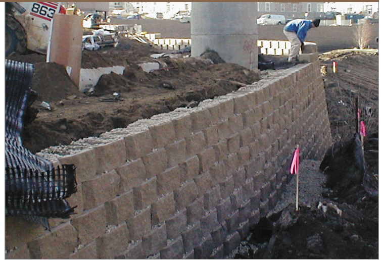
The Diamond Pro® retaining wall system was constructed close to building foundations, utilities and drop structures, like this storm water drain.
