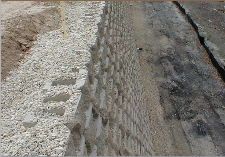
During Phase 2 of the project, the wall was constructed within 10 feet of a stream. Based on global-stability studies performed for the wall in the area near the stream, the wall designer compensated for the reduced strength of the submerged foundation soils.
